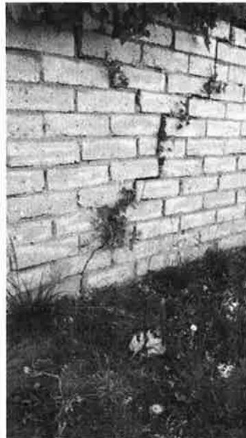
Major crack in wall by tree 4
