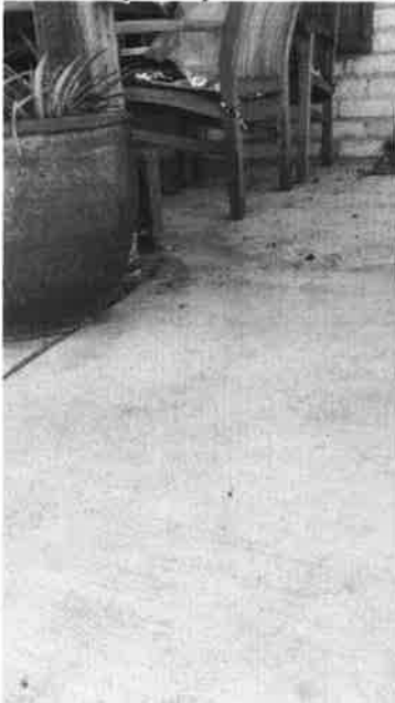
Expansion crack near chair legs
