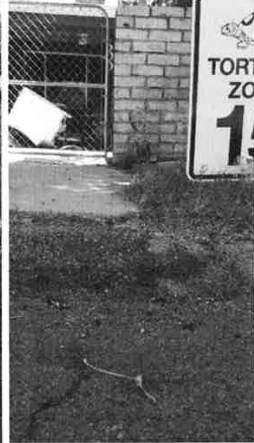
Side walk not raised on tree side
