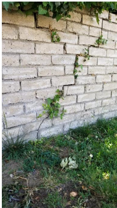
Major crack in wall by tree 4
