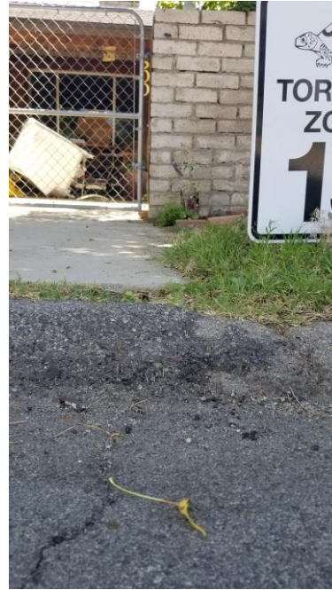
Side walk not raised on tree side
