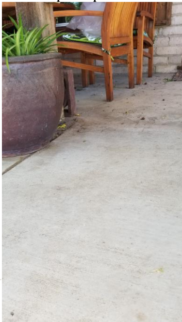
Expansion crack near chair legs
