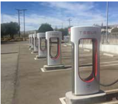
A state of the art charging station near Inyokern
