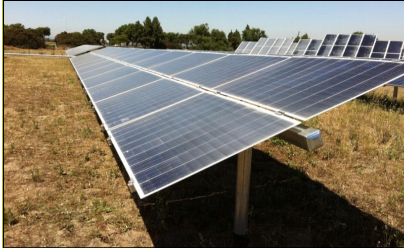
Typical single-axis tracking solar panels
