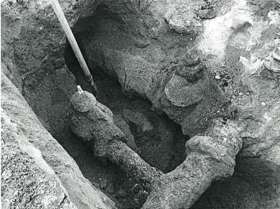
Photo 1 – 6-inch Blind Flanged stub welded to the 8" main at the corner of Locust Street and Mount Whitney Drive, note water below from leaking pipes and joints. This stub was not able to be clamped, 10-mil plumbers tape was wrapped around the entire stub to minimize the leak and then re-buried.
