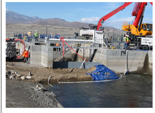
View from rail car bridge at the downstream coffer dam. The lower 225 LF of tailrace channel below the LG is filled 3 to 4 Ft. deep with sands and river sediments. This needs to be cleaned also.
