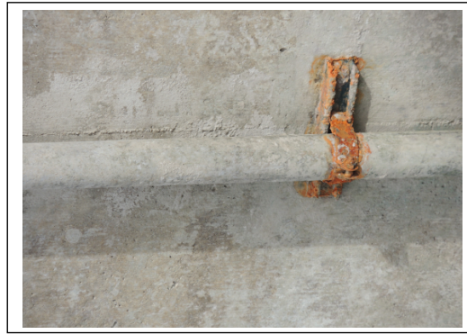
The communication pipe is A304 stainless steel, but the Uni-strut wall straps were only galvanized steel. All three wall brackets need to be replaced with A316 Stainless steel uni-strut and bolting.
