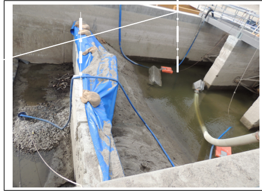
Crews installed concrete barrier blocks and tarp D/S of the three radial gates to prevent inflows from the 3 leaking radial gates tarped, but never sealed.
