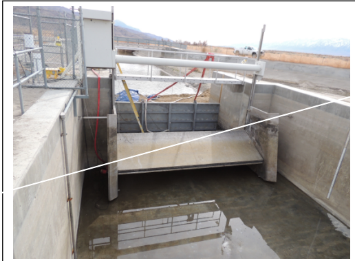
View of the cleaned and pressure-washed Langemann Gate ready for inspection . Note the downstream bulkhead gate and the dirt coffer dam preventing the river from flowing back into the sand trap.
