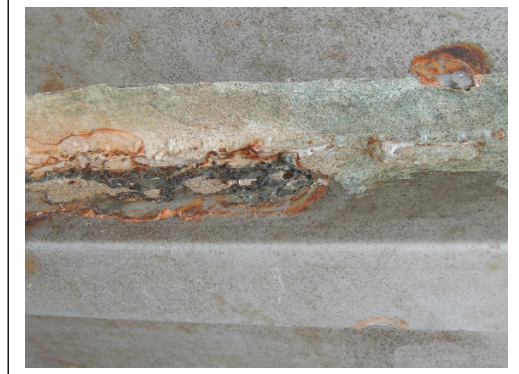
Typical rust-through holes in both of the original gate side plates. A quote of $ 9,900 dollars was received in 2016 for new side plates constructed of A316 corrosion-resistant Stainless Steel.
