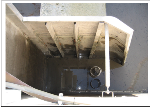
Top view of a LG side plate with stand-off bar. Although the LG was constructed of A304 stainless steel, the thin side plate metals were only plated stainless steel which corroded at seams & welds.
