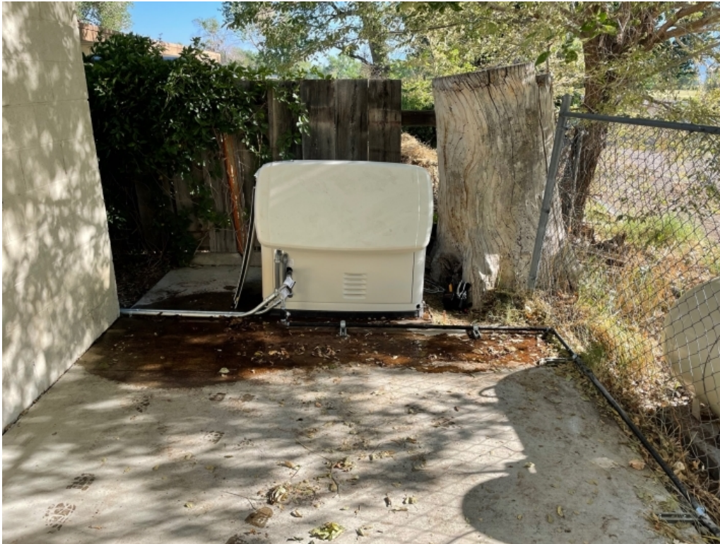
Progress House Generator
