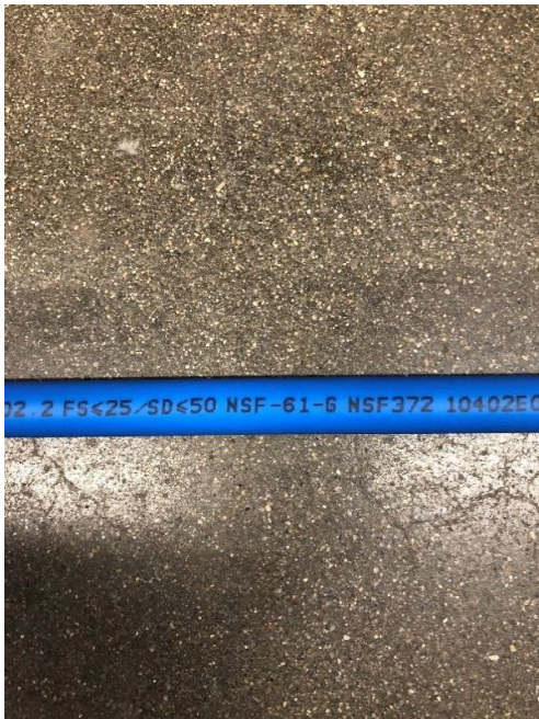
Blue potable PEX line with NSF label
