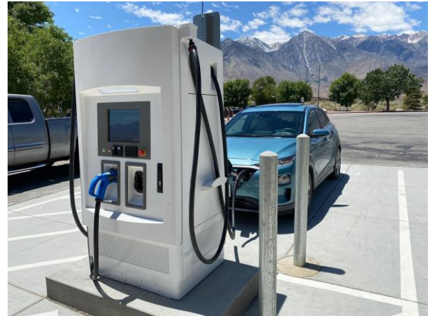
FIGURE 6: DCFC AT HIGHWAY REST STOP
