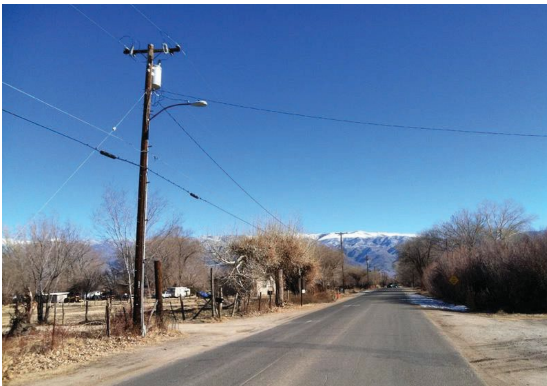
Typical Pole Mounted Street Light on Diaz Lane
