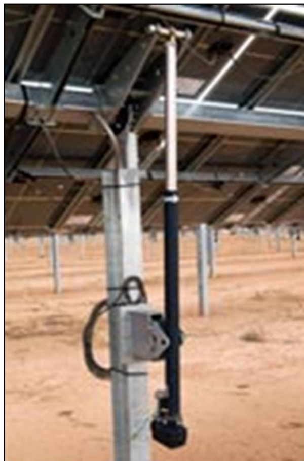
Figure 7-2. Solar Tracker and Actuator
