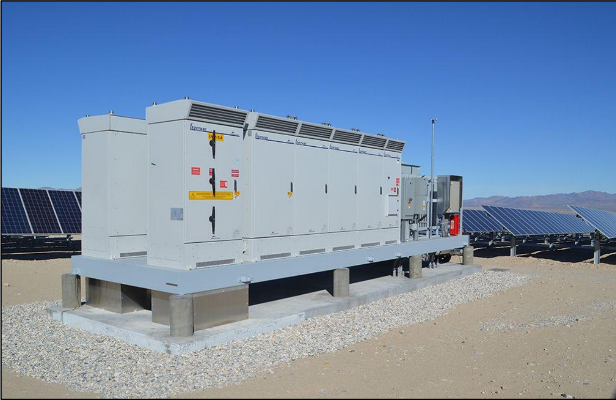
Figure 7-6. Typical Inverter Station
