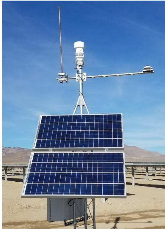
Figure 7-8. MET Station (Photo: Nor-Cal Controls 2024)
