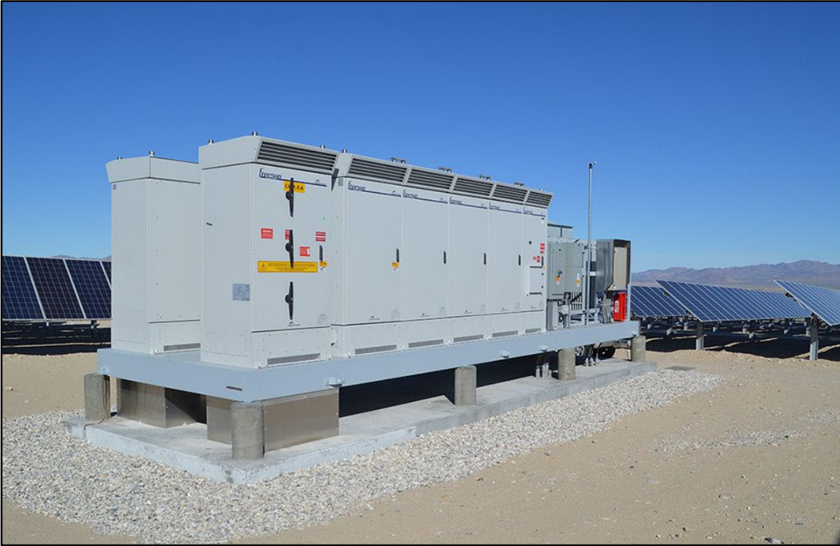
Figure 7-6. Typical Inverter Station
