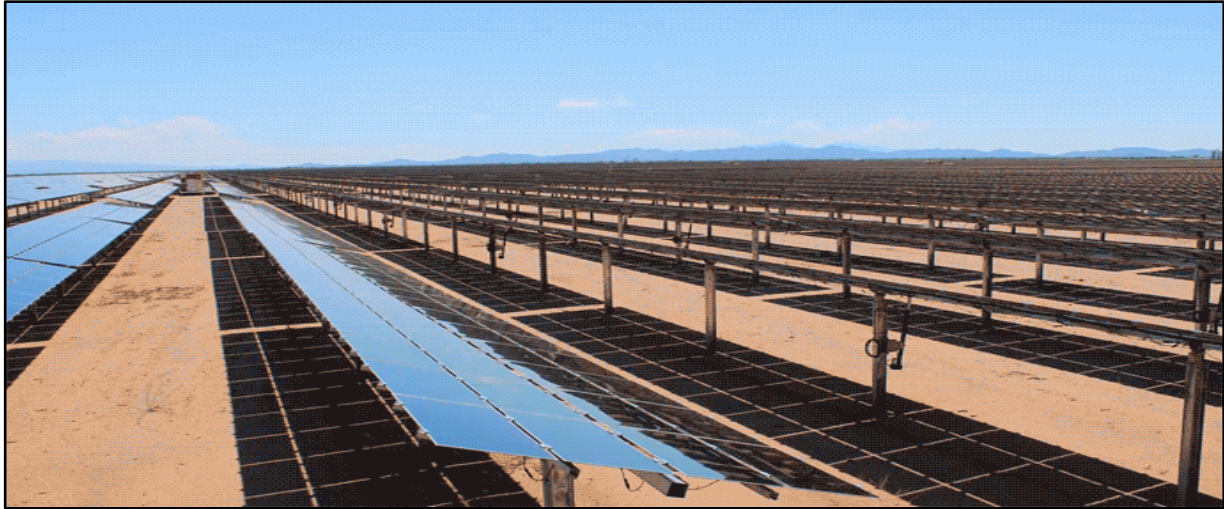
Figure 7-3. PV Module Tracking
