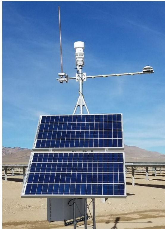
Figure 7-8. MET Station (Photo: Nor-Cal Controls 2024)
