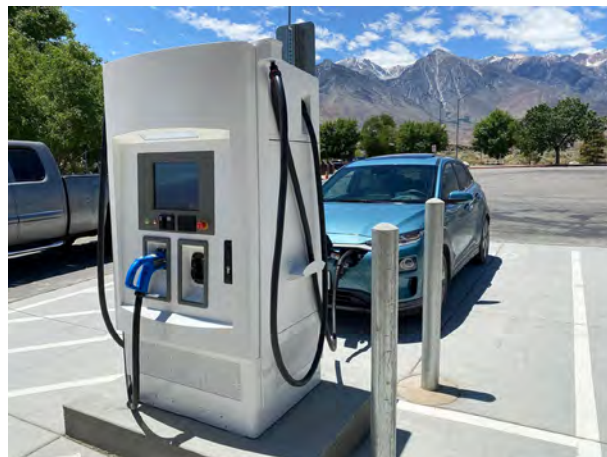
FIGURE 6: DCFC AT HIGHWAY REST STOP
