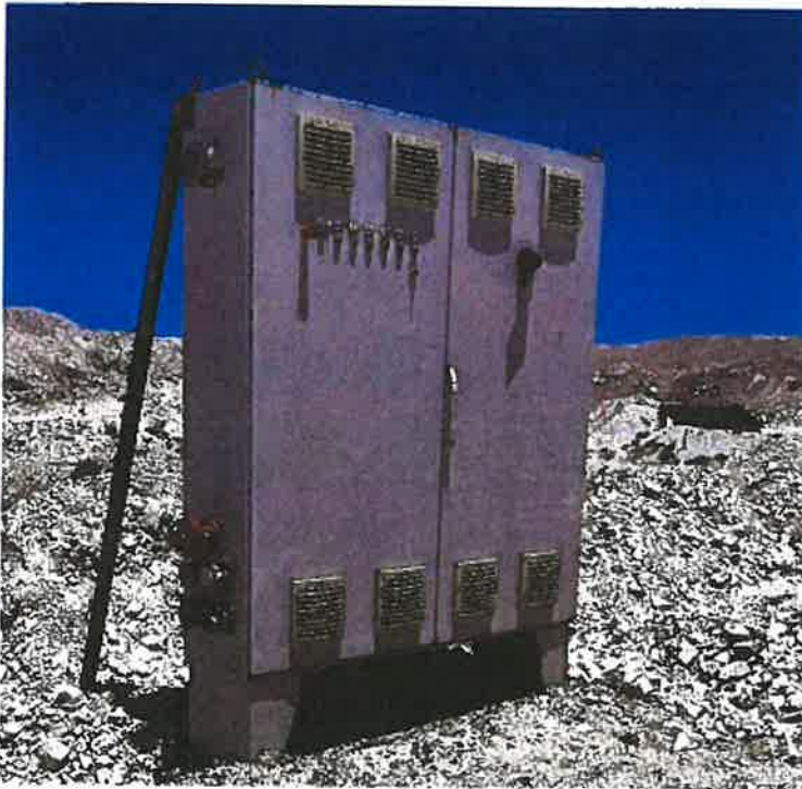
V to E of electrical panel for portable generator and jaw crusher
