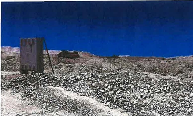
V to N of electrical panel, Sany SY 500 excavator and Sany 405K front-end loader
